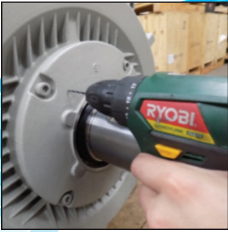
9) Drill hole with 2.5mm Steel drill bit. **NB Caution - Drill to 4mm Depth only.
