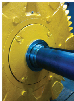
224 kw Motor from the Illovo Group with Earthrings.
